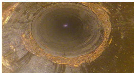
Internal Plastic Coating Condition 2
