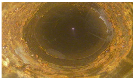
Internal Plastic Coating Condition 4
