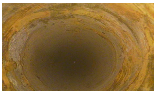
Internal Plastic Coating Condition 3
